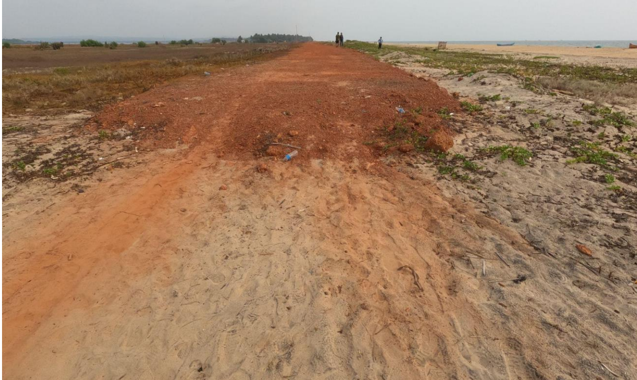
Figure 4: Halted Road Construction
