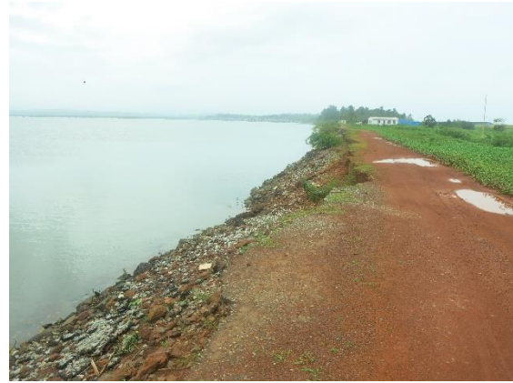
b. Erosion along the eastern boundary of the proposed site
